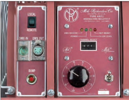
Close-up of Control Panel
